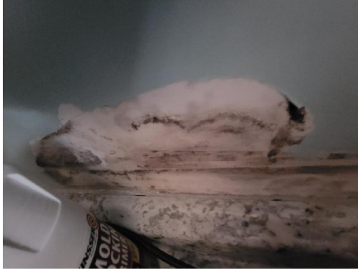
Interior Kitchen Northeast drywall wall Visible water damage Visible microbial growth
